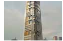
Gate Tower, Sharjah, UAE (Marley)
