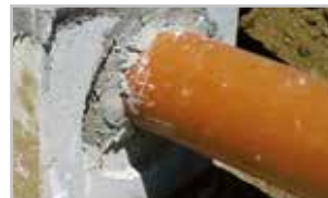
Leakage (in the long term)
